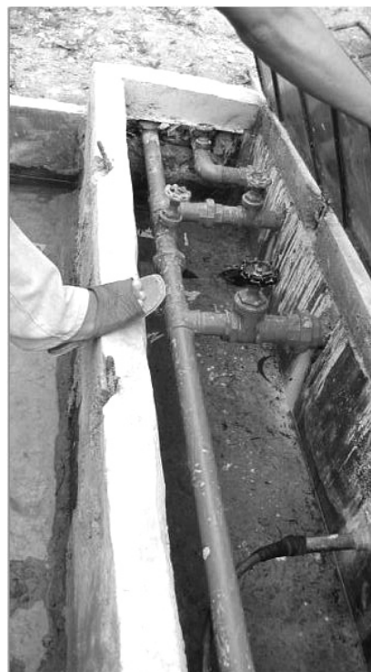
Plumbing fixtures of a ferrocement tank, Nagkahiusang Mag-uuma sa Overland (NAMAQ), Brgy. Overland, Buenavista, Bohol
