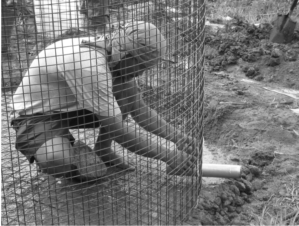
Installing plumbing fixtures to the frame of the ferrocement tank, Bgy., Sirao, Cebu City
